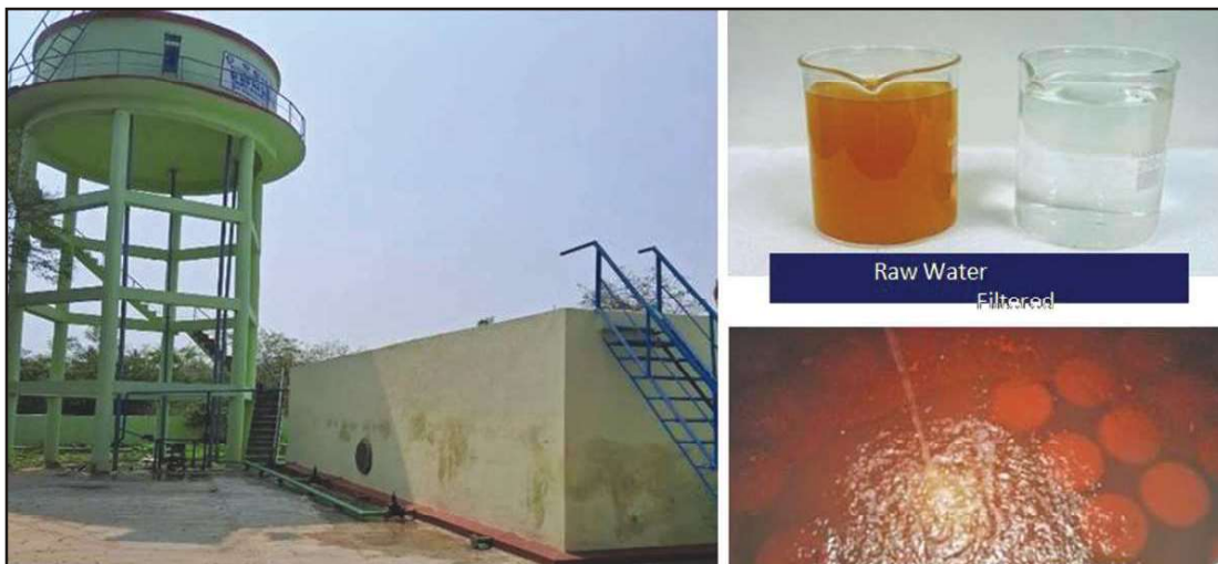
Fig 8. (a) 60KL/day TERAFIL Filter plant; (b) Source water inside TERAFIL Plant with filter media; (c) Raw water and product water quality.
