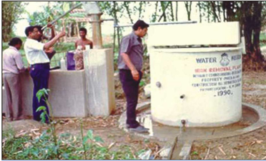
NEERI's hand pump attachable Iron Removal Plant in Assam
