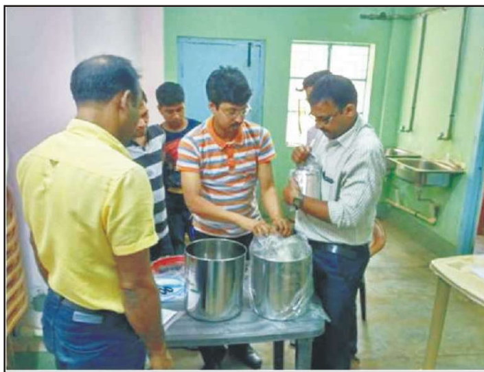
Installation of domestic water filter (defluoridation) at the Office of CMOH, Suri, Birbhum district, West Bengal
