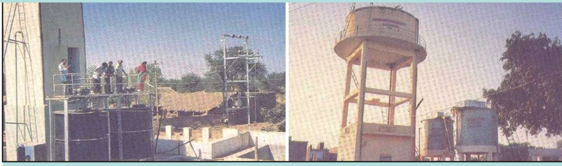
Fill-and-draw Defluoridation Plant at Badarpur, Gujarat
