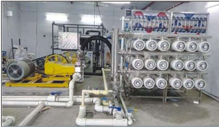
The pilot plant membrane rejuvenation facility at CSIR-CSMCRI ESF
