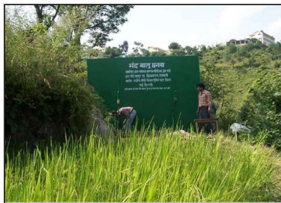
Slow Sand Filters designed, constructed and commissioned by NEERI at village Chhati in hilly region of Tehri Garhwal
